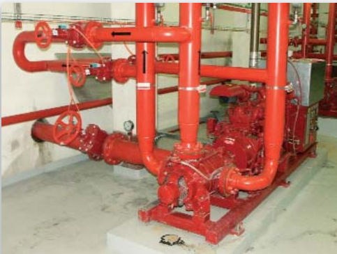
Typical Multi Stage Pump Installation (Motokov building in Prague)
